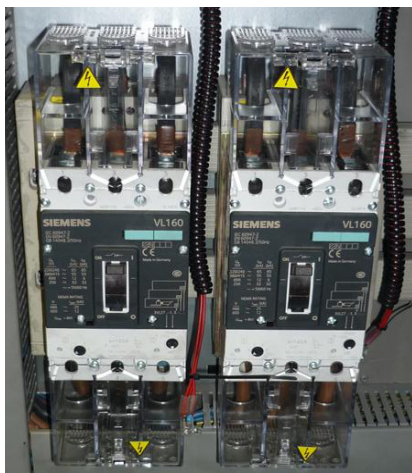
After the replacement, the first section consists of the actual circuit breakers.
