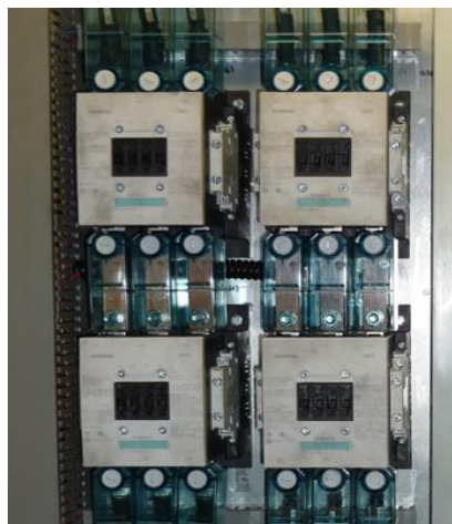
After the replacement, the second section consists of contactors to power linear motors and inductions.
